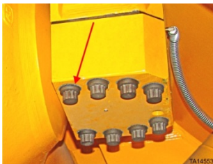
Arrow indicates location to be cleaned
